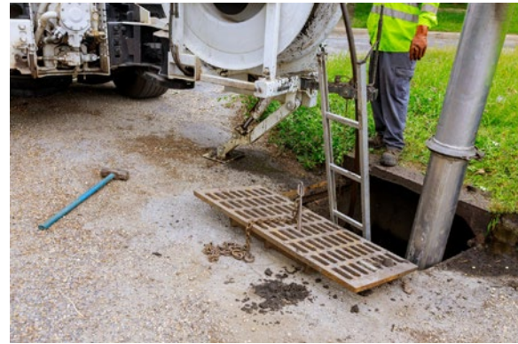
▲ Cleaning out catch basins is important to ensure proper drainage (photo by Mr G’s Excavation & Grading, licensed by CC BY-NC 4.0)
