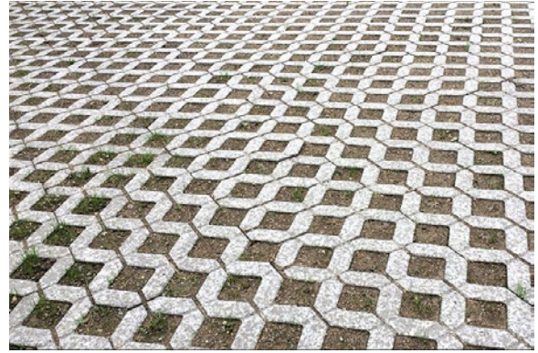
▲ A driveway made of permeable pavers, which, when maintained properly, reduce stormwater runoff by allowing it to infiltrate the soil
